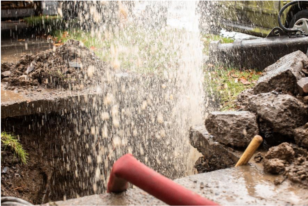
Example of leakage
