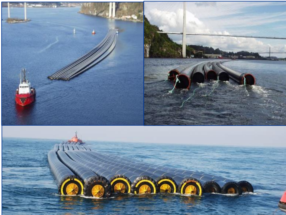
Figure 33: Transport of Long Lengths of Pipe to Site – copyright PipeLife Norge AS
