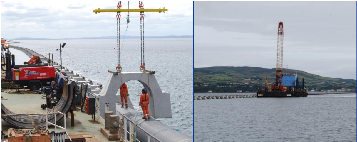
Figure 36: Concrete Ballast and pipe assembly being installed on floating pipe in sheltered water
