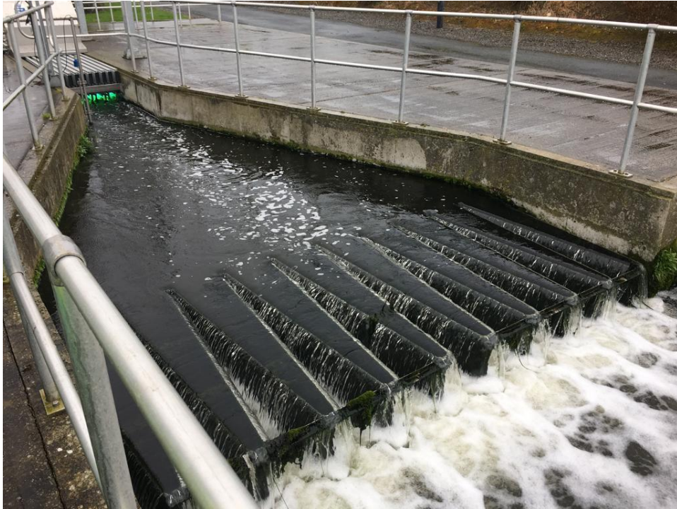
Figure 1 Photograph showing Irish Water UV disinfection system at a WWTP
