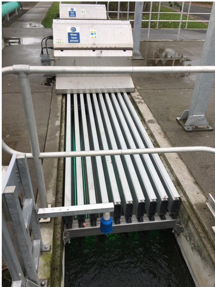
Figure 2 Photograph of module of UV lights installed in a channel at Irish Water WwTp
