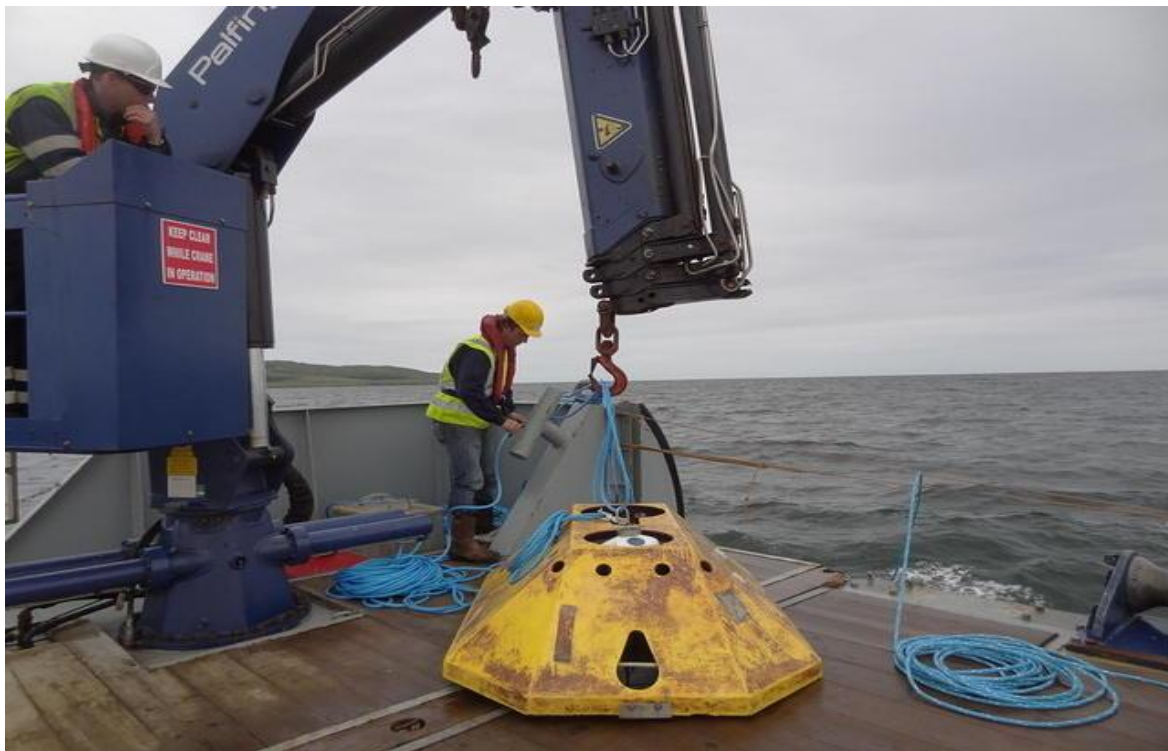
Figure 6. The deck crane being used to lift the AWAC trawl-resistant frame into the water
