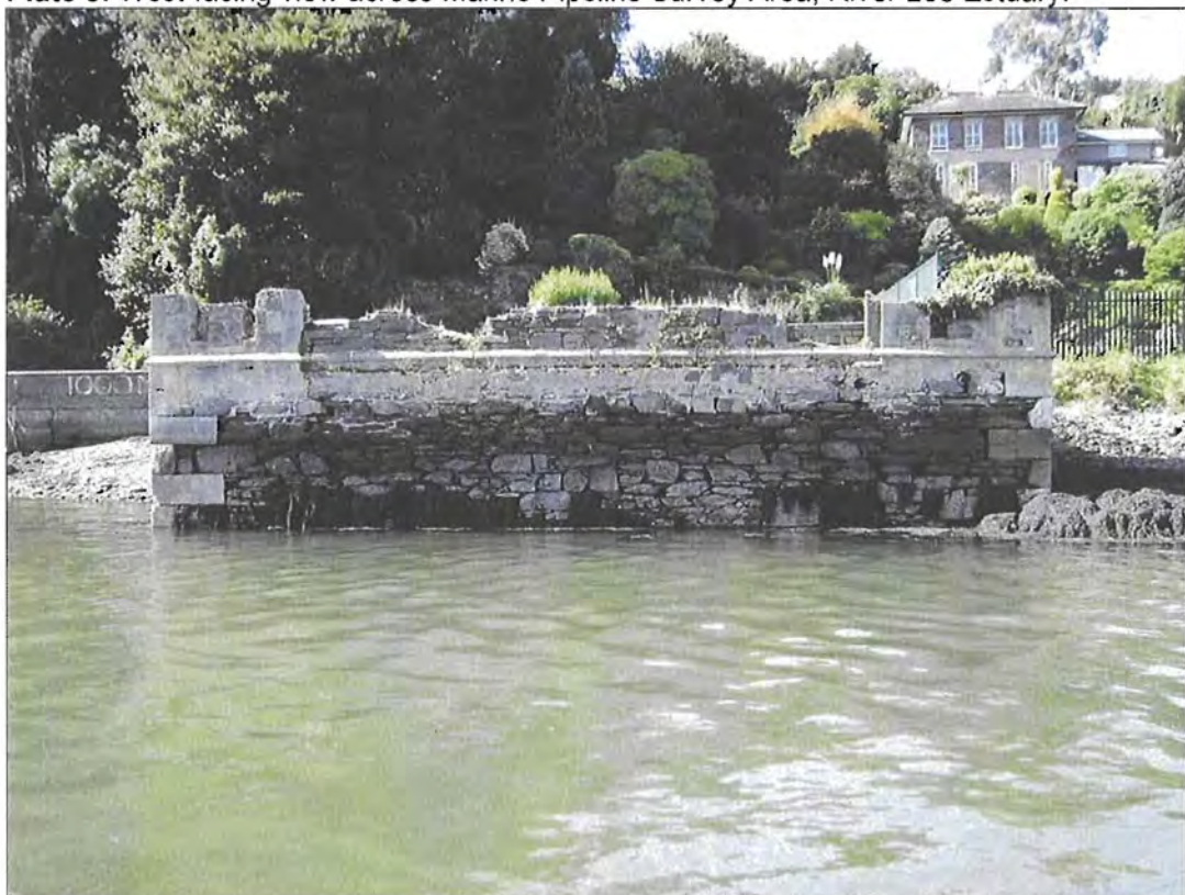
Plate 4: West-facing view of downstream (southern wing) masonry façade from the remains of the Royal Victoria Baths located on the west side of the River Lee.
