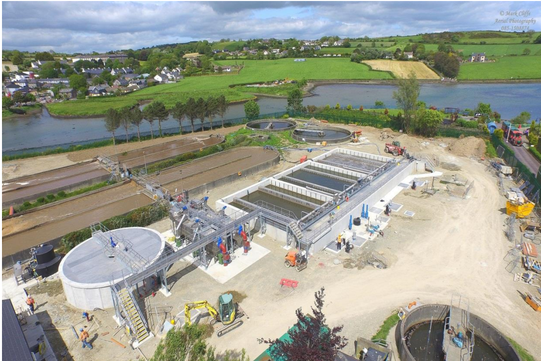
Figure 5.2 – Clonakilty Wastewater Treatment Plant
