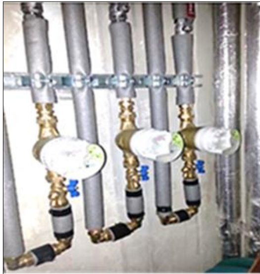
Photo 2: Example of pipe inserts looped down from ceiling to install meters at eye level
