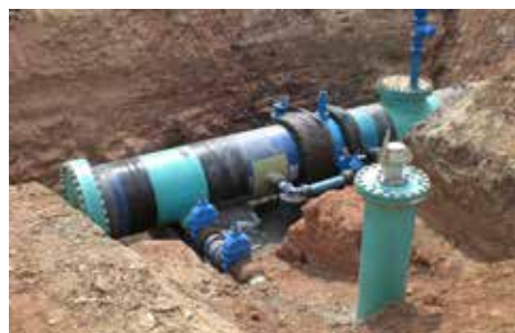
Example of below ground valves
