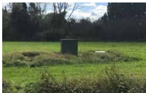
Example of a valve control kiosk
