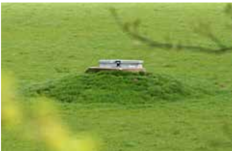
Example of a typical air valve
