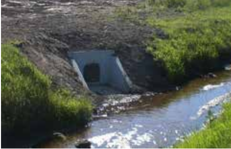
Example of a washout
