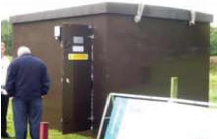
Figure 6: Typical orthophosphate dosing unit
