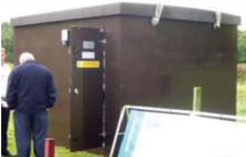
Figure 3 Typical orthophosphate dosing unit
