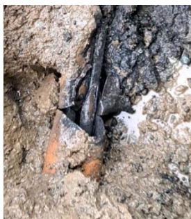
Photo1: Pipe & Cable post incident
