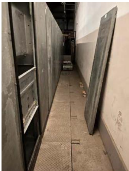
Picture 1: Main intake substation
