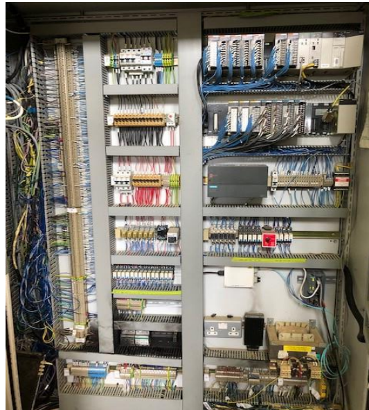
Picture 1: Panel Before works commenced
