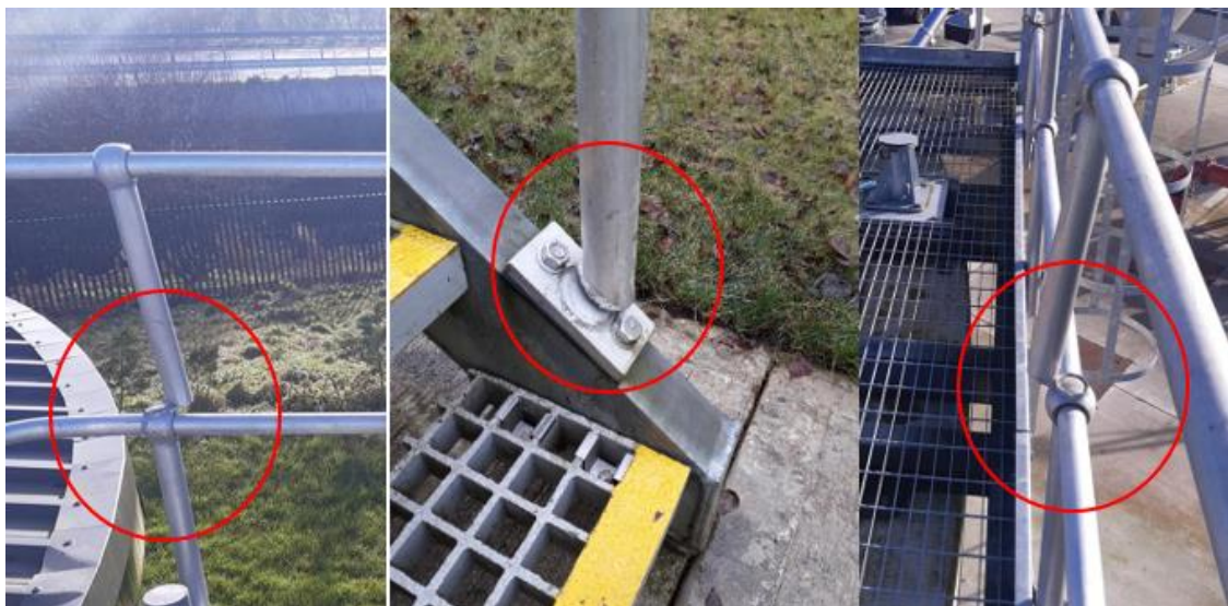
Picture 1: Weld Failures on Stanchions
