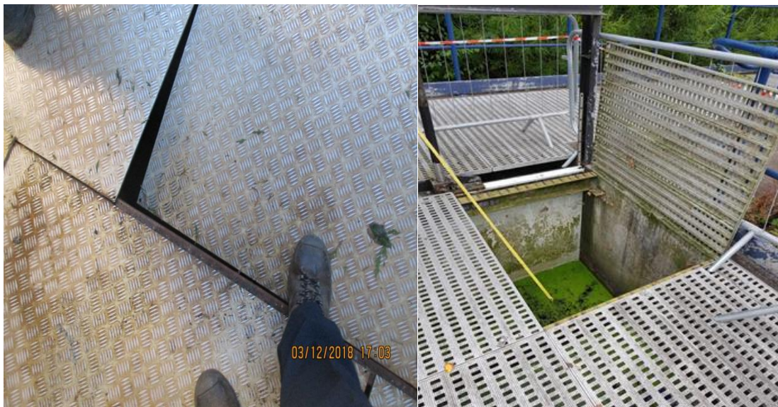
Photo 1: Checker plates & Grid Flooring
