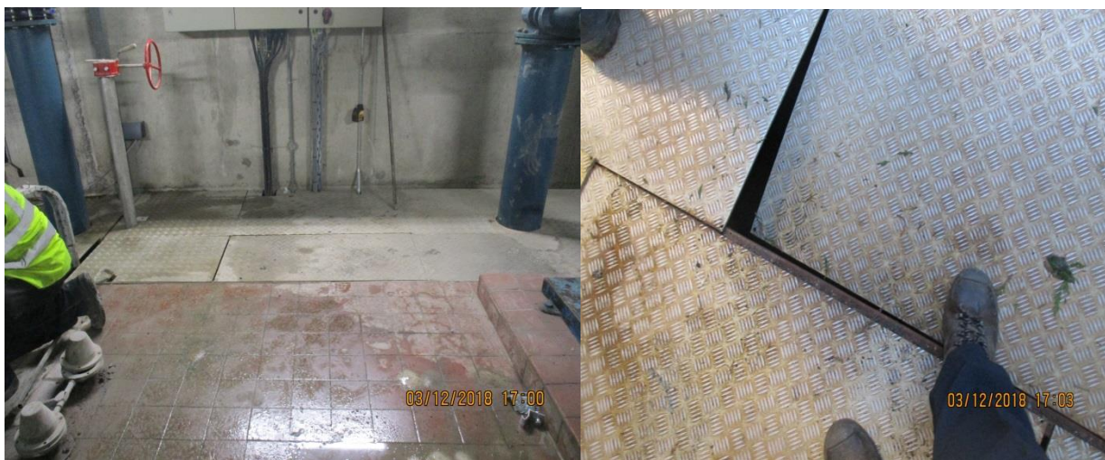
Photo 1: Checker plates where incident occurred
