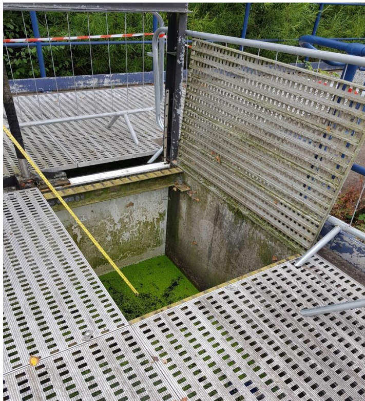
Photo 1: Grid flooring over Inlet Works
