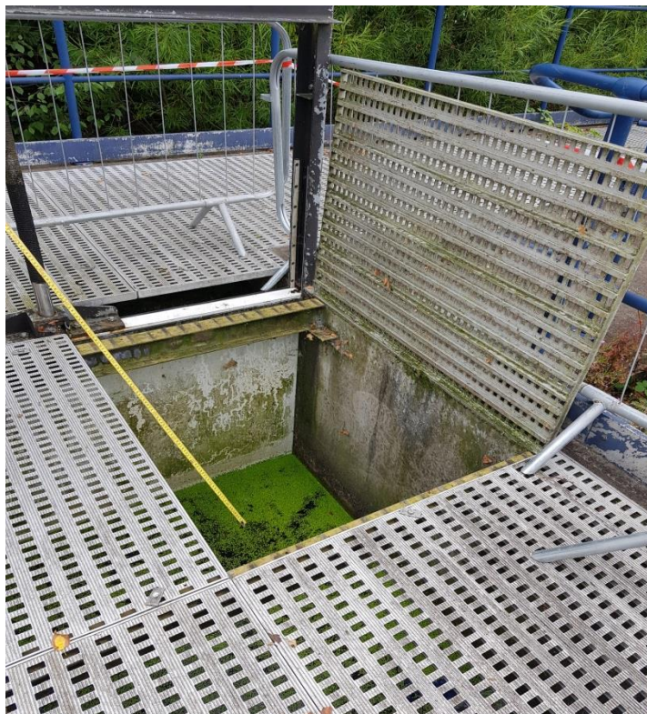
Photo 1: Grid flooring over Inlet Works
